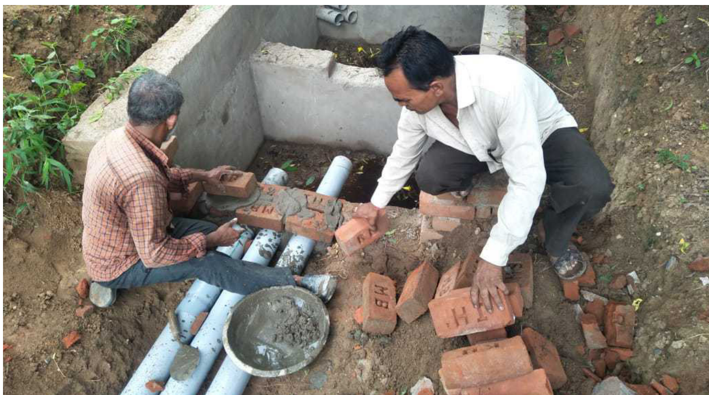
Two men build a rainwater harvesting structure. Inspired by the work and commitment of Lokmitras, the State Bank of India committed Rs. 2.5 million for water harvesting in one of their villages.
