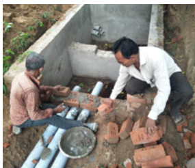
Two men build a rainwater harvesting structure. Inspired by the work and commitment of Lokmitras, the State Bank of India committed Rs. 2.5 million for water harvesting in one of their villages.
